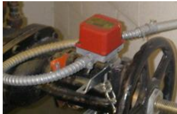
Tamper switch on a sprinkler valve
